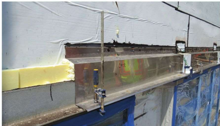
Creating a continuous air barrier from the wall to the shelf angle with a stainless steel flashing. The author also installed a spray polyurethane foam (SPF) solid under the stainless steel flashing to reduce the condensation potential under the flashing.
