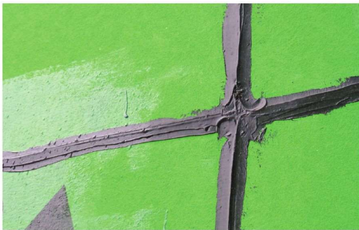
Proper sheathing joint detailing (approximately 3.2 mm [0.125 in.] thick by 25 mm [1 in.] wide approved joint material with proper water shedding slopes.
