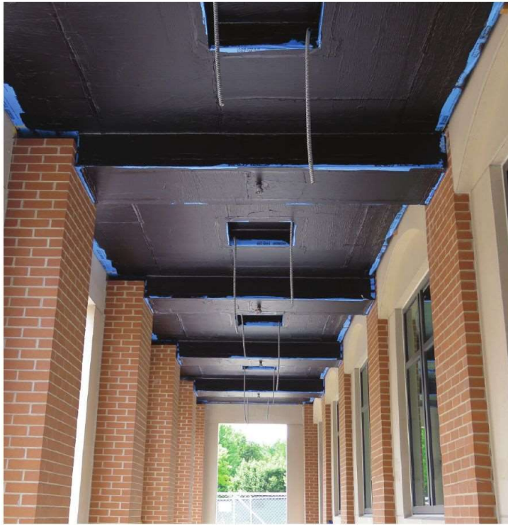
Upper soffit for the air barrier, including the electrical lightbox. A finish soffit will be installed under this soffit.
